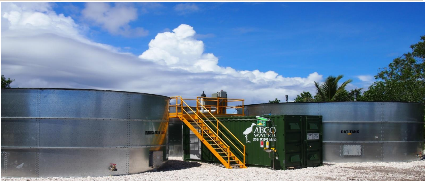
1400EP Waste Water Treatment Plant in Nauru
