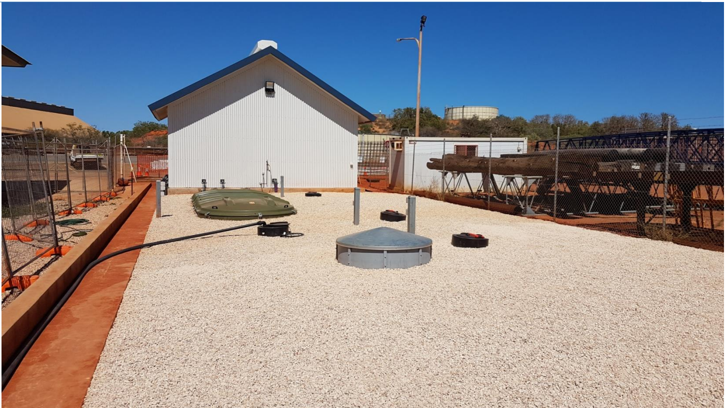
Vacuum Collection & RBC Waste Water Treatment Plant (RWQMP Compliant) Complete with Cyclone rated Building housing the Control room and equipment
