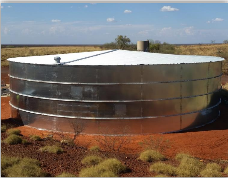
Recently Installed 1000kL Storage Tank
