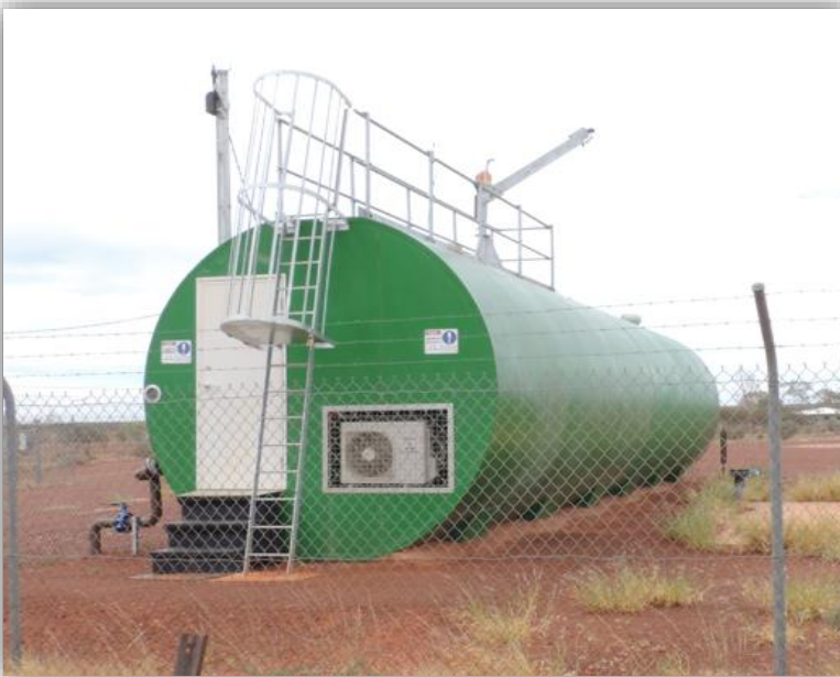
105kL Water Storage and Pump Room
